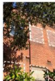
Filled in windows reopened with original facade openings restored, and signage repaired
